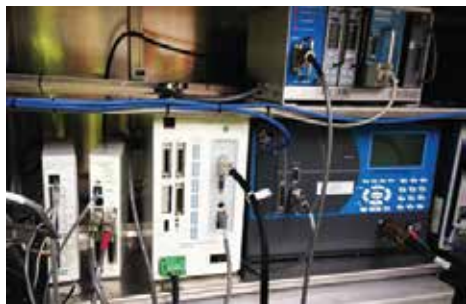
Adaptive Signal Control Equipment
